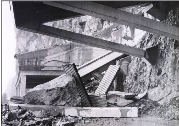
Fig. 1: Gallery destroyed by rockfall event (500-600 m 3 ) in 1970.
